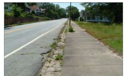
Above: Sidewalk maintenance needed on Montgomery Ave
